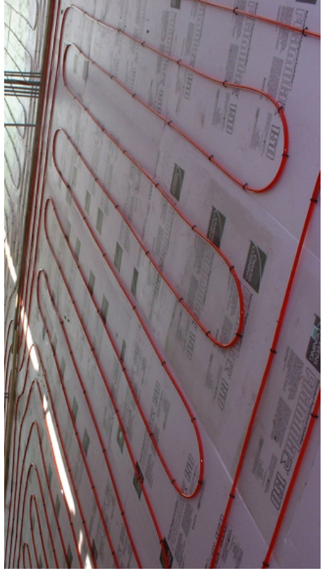
Wall mounted radiant panels
